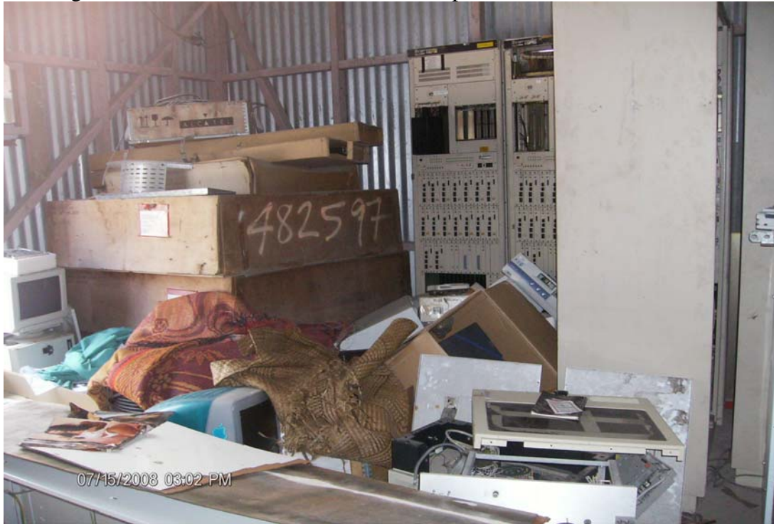
Figure 11 Couple of DRCS at TSKL Storeroom
