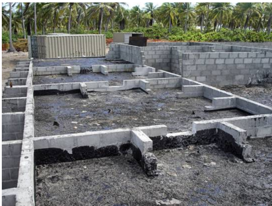
Fig. 3. The Bitumen Processing Area that allowed for the recovery and recycling of bitumen.
