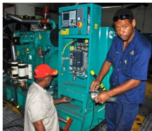
Biofuel Generator Installation Solomons
